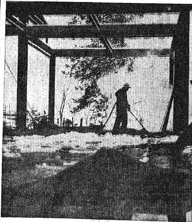
ABOVE: "Neither sleet nor snow . . ." A workman pushes snow from the half-finished floor. During the winter the workmen were protected from the weather by plastic sheets attached to the scaffolding.
